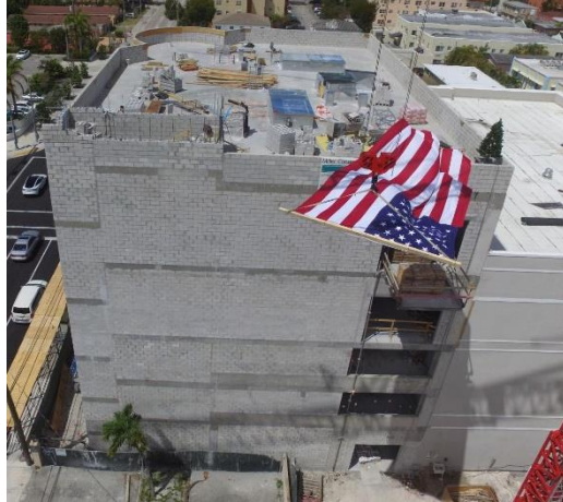
"Topping-Out" Tradition: American Flag and pine tree placed on top of the 5th story of Miami Lighthouse Classroom Expansion.
